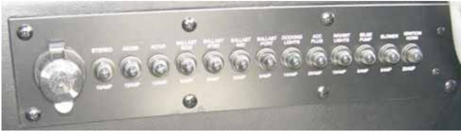
Figure 2-4. Circuit Breaker Panels
