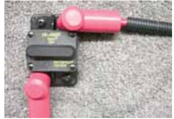
Figure 4-4. Main Circuit Breaker
