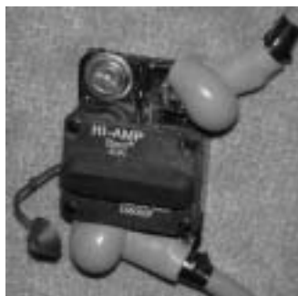
Figure 4-2. Main Circuit Breaker
