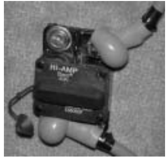
Figure 4-3. Main Circuit Breaker
