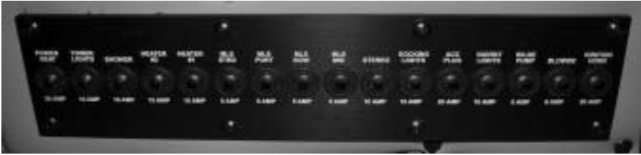
Figure 2-7. Circuit Breaker Panel
