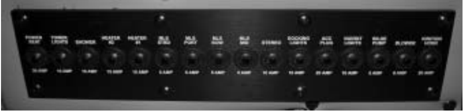
Figure 2-12. Circuit Breaker Panel
