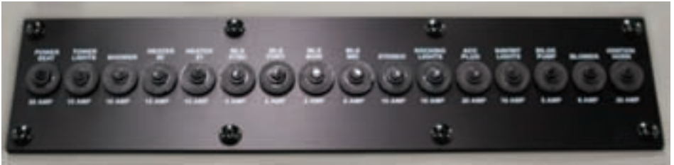
Figure 2-9. Circuit Breaker Panel
