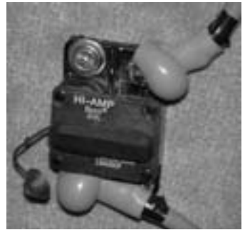
Figure 4-3. Main Circuit Breaker
