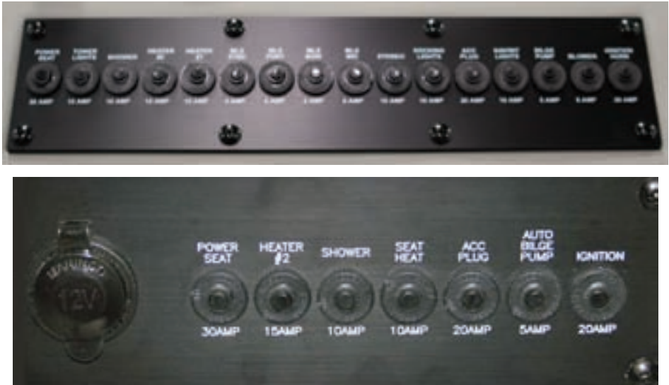
Figure 2-9. Circuit Breaker Panels
