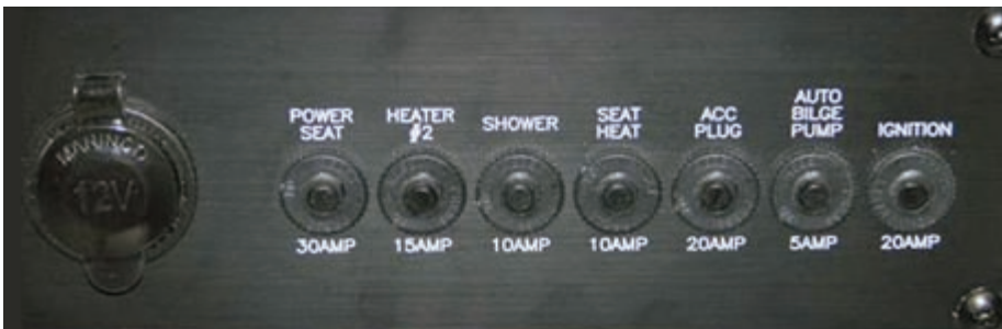
Figure 2-13. Circuit Breaker Panels
