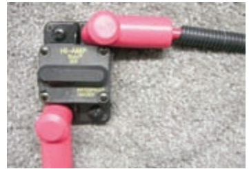
Figure 4-8. Main Circuit Breaker
