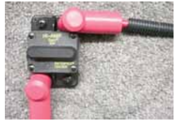
Figure 4-12. Main Circuit Breaker
