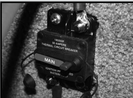
Main Dash Power-Circuit Breaker
