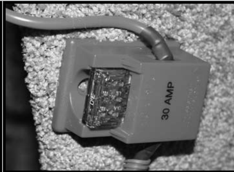
Fuse Panel - Battery Connection
