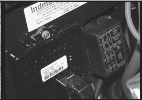
Fuse Panel - Back of Engine
