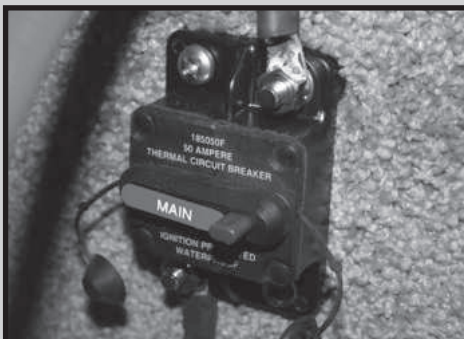
Main Dash Power-Circuit Breaker
