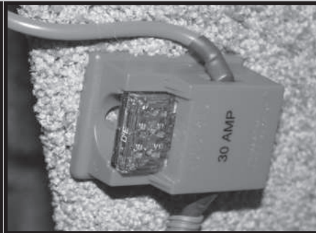
Fuse Panel - Battery Connection
